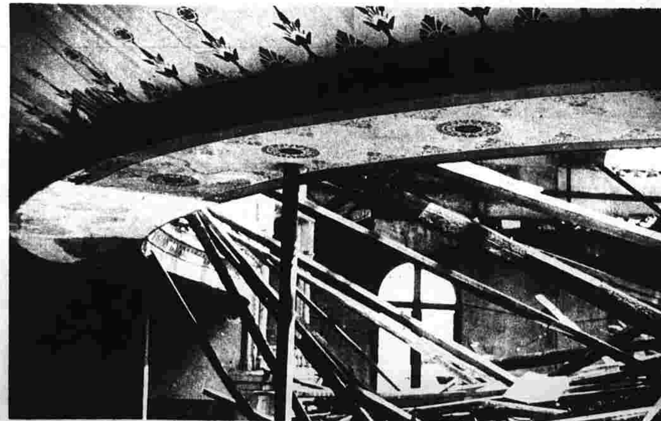
Ceiling of horseshoe-shaped balcony of the old Henry Opera House on the third floor. Operettas were performed there.
